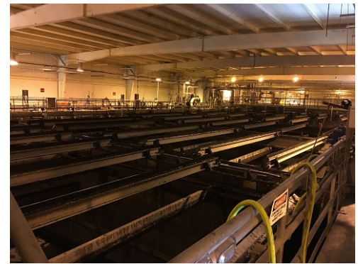
Adams Street WWTW PURAC Filter Cells
