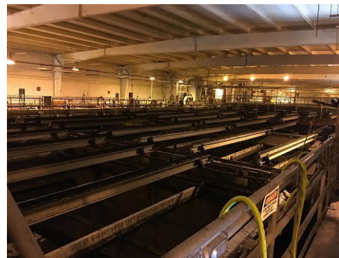
Adams Street WWTP PURAC Filter Cells
