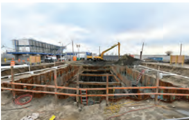
South stormwater pump station
