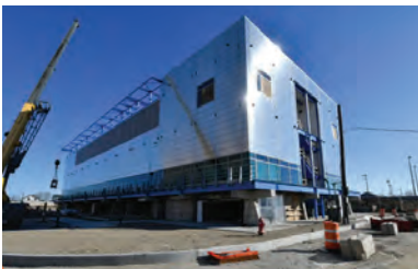
New electrical substation
