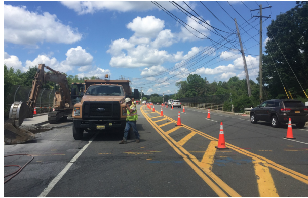
Traffic Control on Design and REI services for Suez Water Main Lining Project, Airmont, NY
