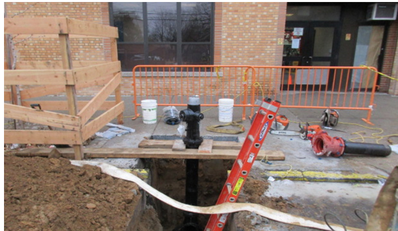
New fire hydrant on the NYCCDC Replacement of Trunk and Distribution Water Mains & Combined Sewer Rehabilitation in Bainbridge Avenue Project
