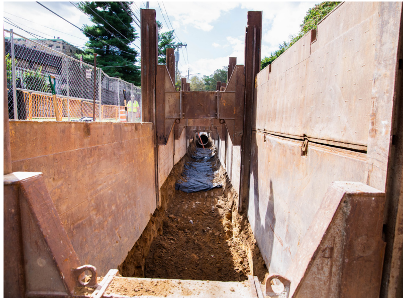
NYCDDC Resident Engineering and Inspection Services for Replacement of Trunk and Distribution Water Mains & Combined Sewer Rehabilitation in Bainbridge Avenue
