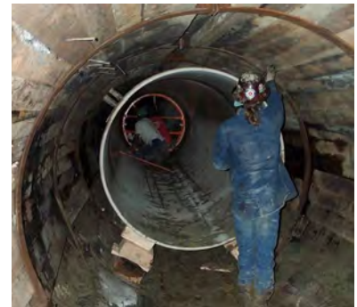
Hazen has extensive experience installing FRP on a variety of projects, and can leverage this experience for NHSA.
