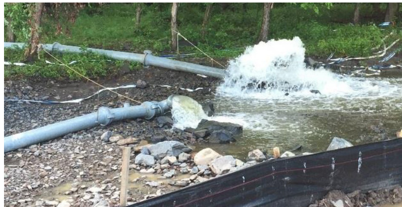
FIGURE 1: BYPASS PUMPING AT THE HORSEPEN DAM ALTERATION (D-B PROJECT ASSOCIATED WITH ROUTE 606 WIDENING), VIRGINIA
