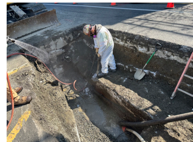
Concrete duct removal for Manhole 280 Expansion. Madison Street Area Infrastructure Improvement, Phase 1
