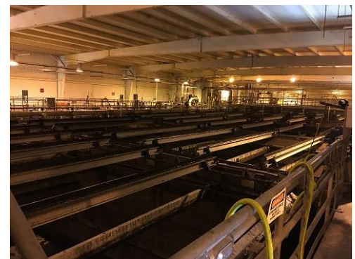
Adams Street WWTP PURAC Filter Cells
