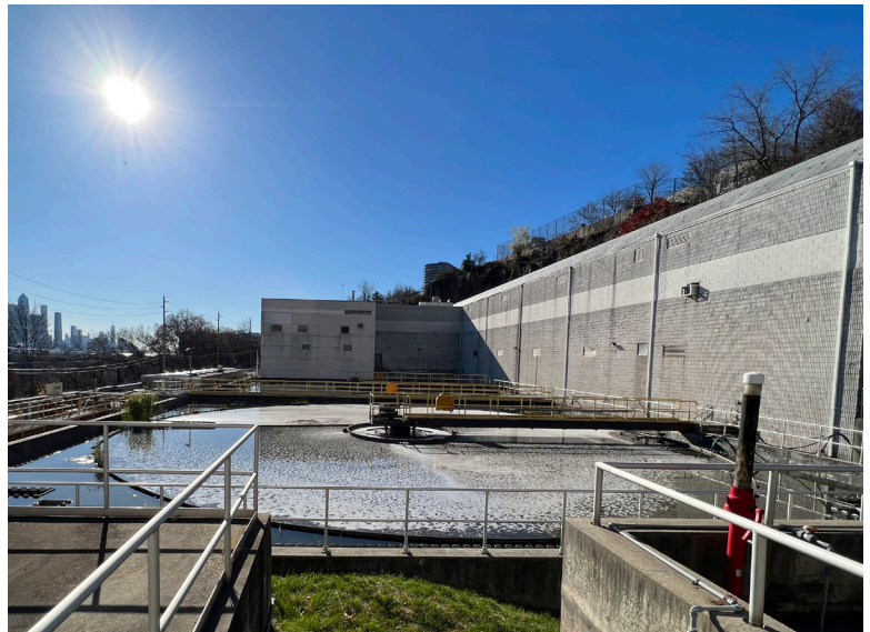
The existing squircle clarifiers at the River Road WWTP, which will need to be demolished and replaced with the high-rate treatment system.
