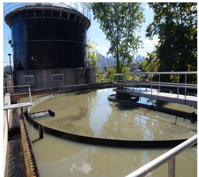
Kleinfelder gained invaluable experience working with NBMUA implementing a membrane treatment system for the direct filtration of trickling filter effluent; including analysis of squircle clarifiers (shown above).
