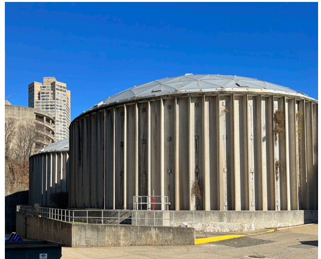
Snails, worms and biofilm sloughing from the existing trickling filters at the River Road WWTP can result in wide fluctuations in TSS concentrations which can adversely impact high-rate treatment systems.
