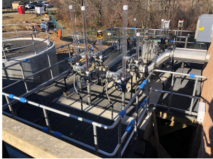
Headworks screening and grit removal facilities.
